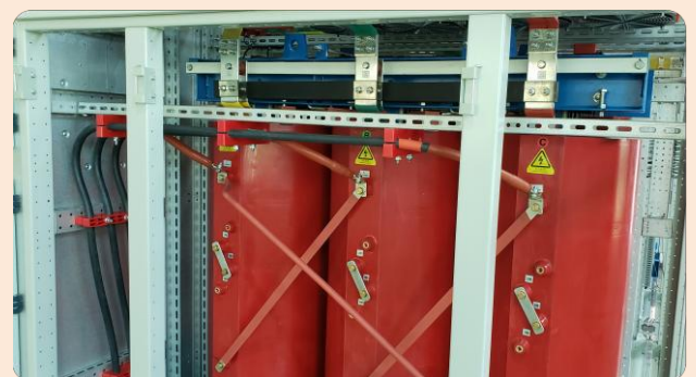
HV / LV Transformers
