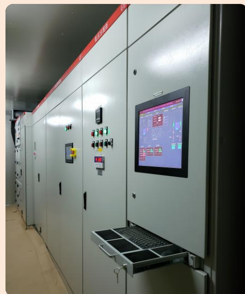
static frequency converter built inside of container
