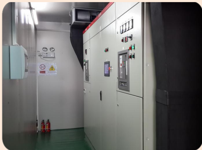
Containerized static frequency container
