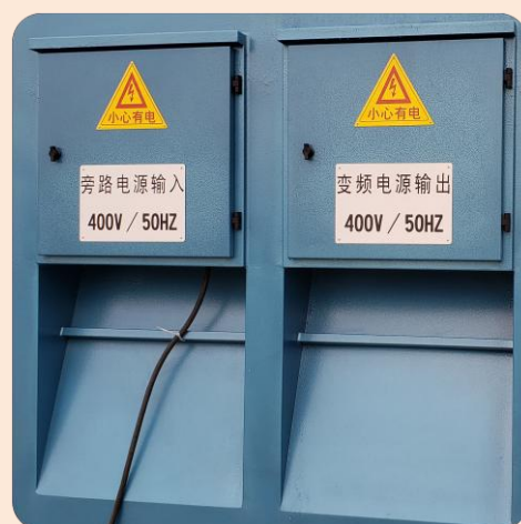
HV/LV cable cabinet
